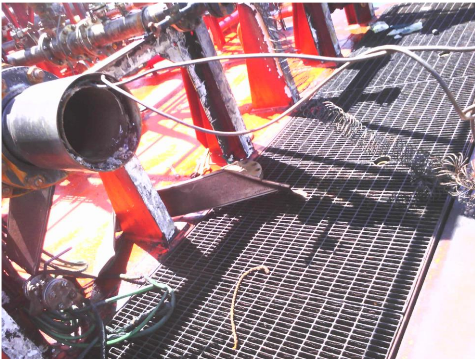
Figure 24: A Snapshot of the Loading-Unloading Hose after Fire Fighting
