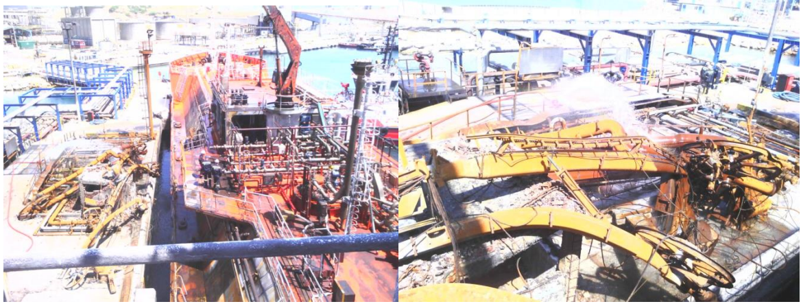
Figure 23: The Snapshots of Berth Damage
